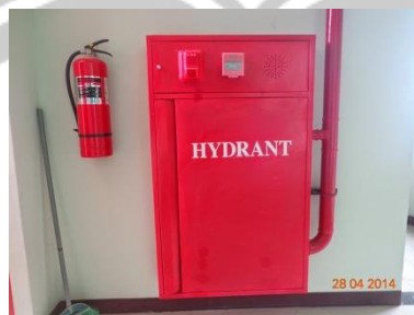
Gambar 6.10 Hydrant (Sumber: www.guardall.com )
