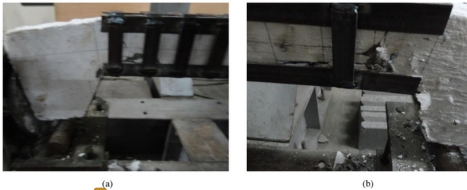
Fig. 6. (a) Crack pattern of the specimen KSV-50; (b) Crack pattern of the specimen KSV-150.
