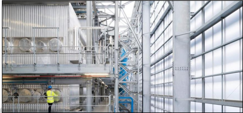
Gambar 2.23 Interior Suffolk energy-from-waste facility
