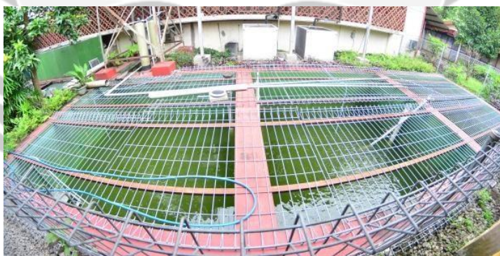
Figure 2.16. Liquid Waste Treatment Area
