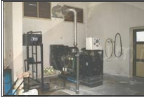
Gambar : 2.57 Ruang Genset Sumber : http://www.pantisemedi.com
