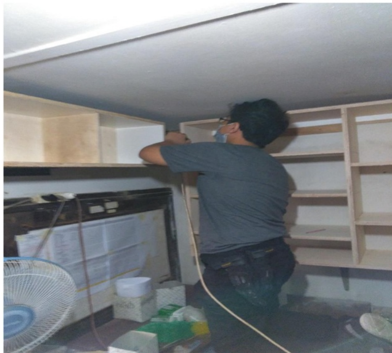
Picture 4.4. New Storage Installation
