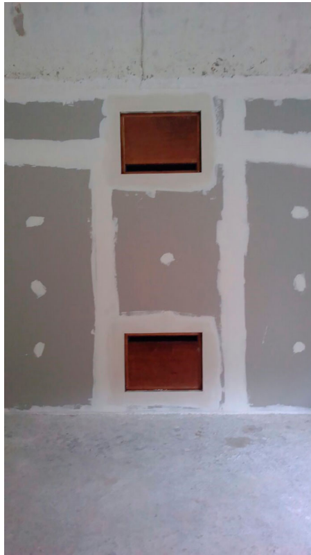
Figure 7. Noise-reducing vents are installed on the soundproof wall of the test chamber (as seen from the sound receiver room). The vents are positioned to simulate their position at upper and lower part of a double-glazed window (which is expected to have an STC of at least 25 dBA, and thus, can reduce outdoor noise from 70 dBA to 45 dBA, as required for indoor noise).
