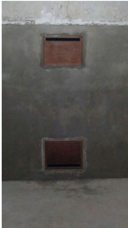
Figure 8. Noise-reducing vents as seen from the sound source room.
