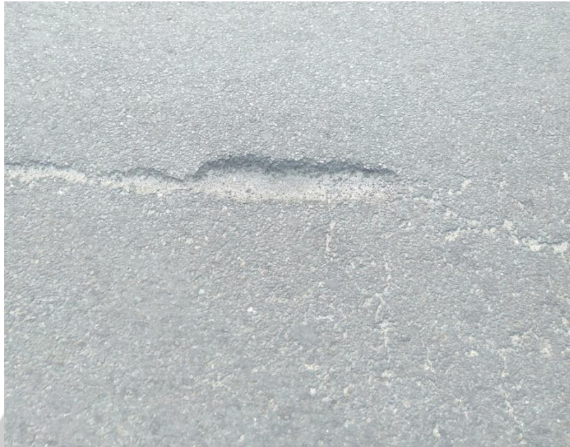
Lampiran C.9 Gambar Kerusakan Lubang
