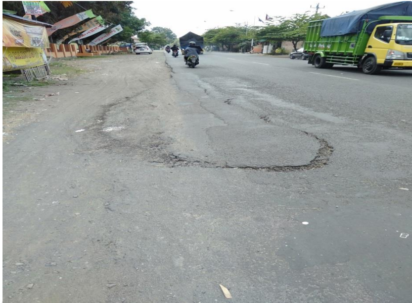
Lampiran C.11 Gambar Kerusakan Sungkur
