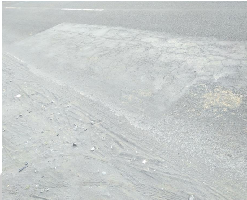
Lampiran C.7 Gambar Kerusakan Tambalan
