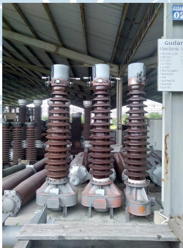
Material Switch Yard Berupa CT 150 kV
