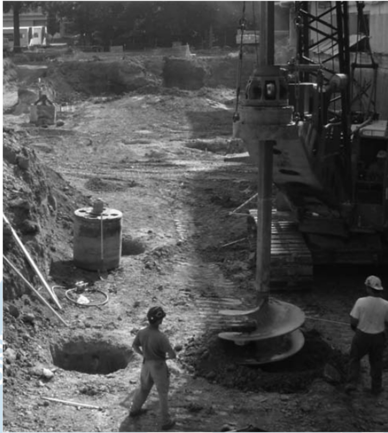
Gambar 3.14 Pekerjaan dengan Metode Kering/ Dry Method (Courtesy of Sanjeev Kumar, Southern Illinois University, Carbondale, Illinois)
