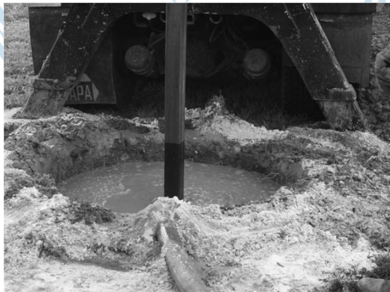
Gambar 3.15 Pekerjaan Bored Pile dengan Metode Adonan/ Washed Boring (Courtesy of Khaled Sobhan, Florida Atlantic University, Boca Raton, Florida)
