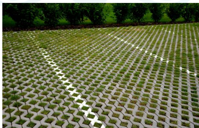
Gambar 3.7.2.4 Sistem Perkerasan Grid Sumber : ( Concrete Grid Pavers Foto Stok, Potret & Gambar Bebas Royalti - IStock , n.d.)
