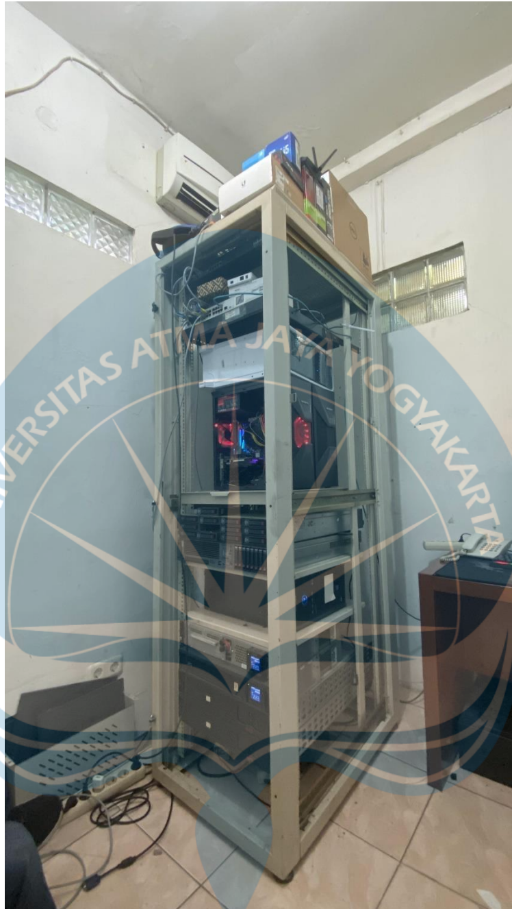
Gambar 7.4. Server Native PT. Central Texindo
