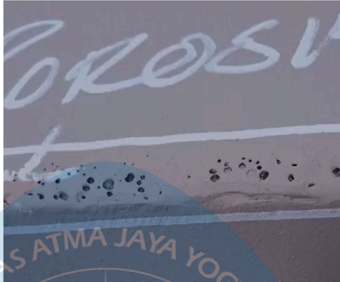
Figure 2.18 Welding Porosity Defect
