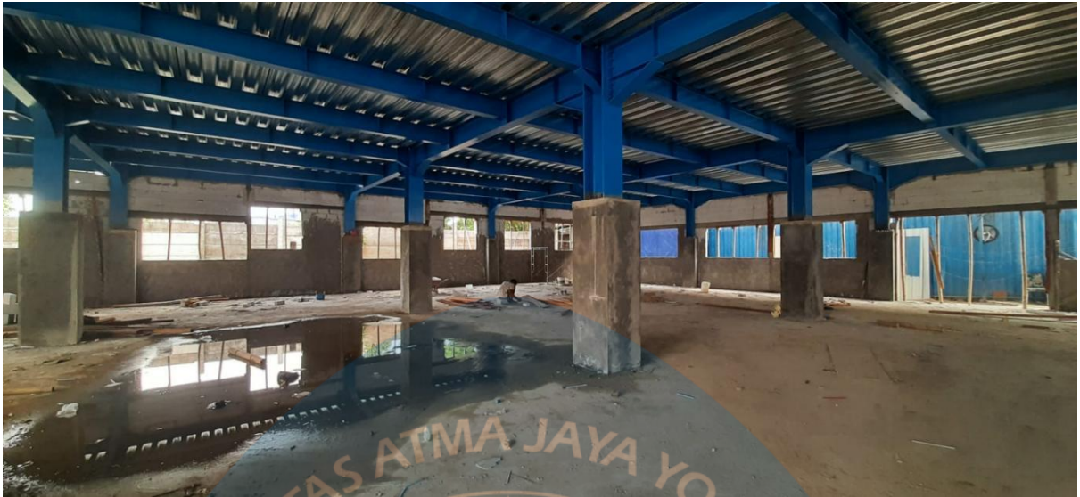
Figure 2.6.12 Condition the first floor after the wall was polish (Clearing area for continue work at the second floor)
